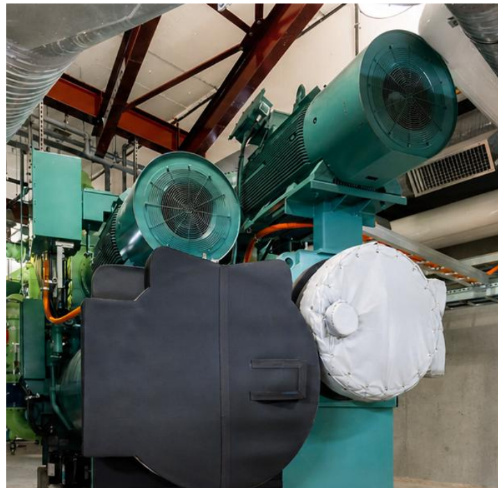
2024 expansion: two 3.3 MW sewage heat pumps
