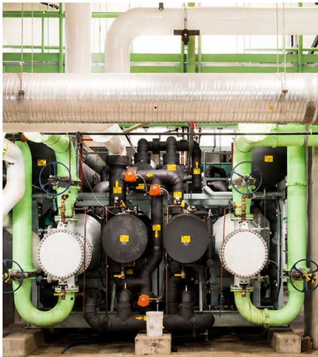
Original 3.2 MW sewage heat pump
